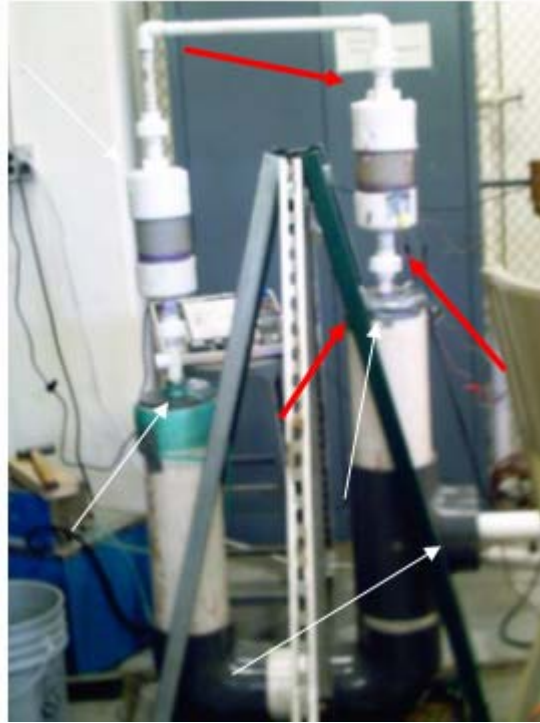
Figure 5.1 Picture of system; the red arrows show where leakage occurred; the white arrow show where frictional losses were observed.
